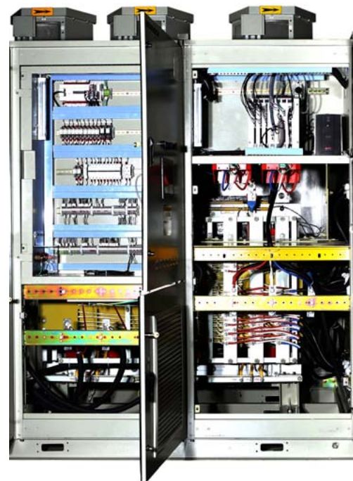
Control- and transformer cabinet
