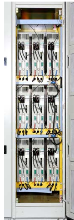
Power cells cabinet
